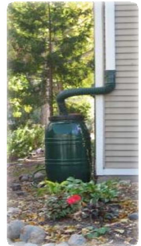
Downspout connection to Rain Barrel
