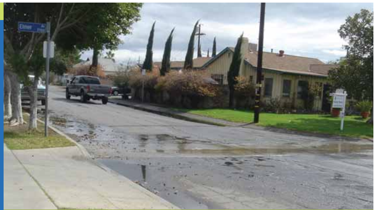
Water accumulates on Elmer Ave. after a rain shower, a problem that will soon be fixed.
