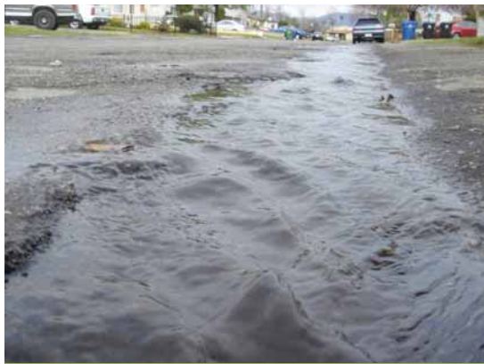
Flooding on Elmer Ave., as shown above, will be contained and managed through various projects.
