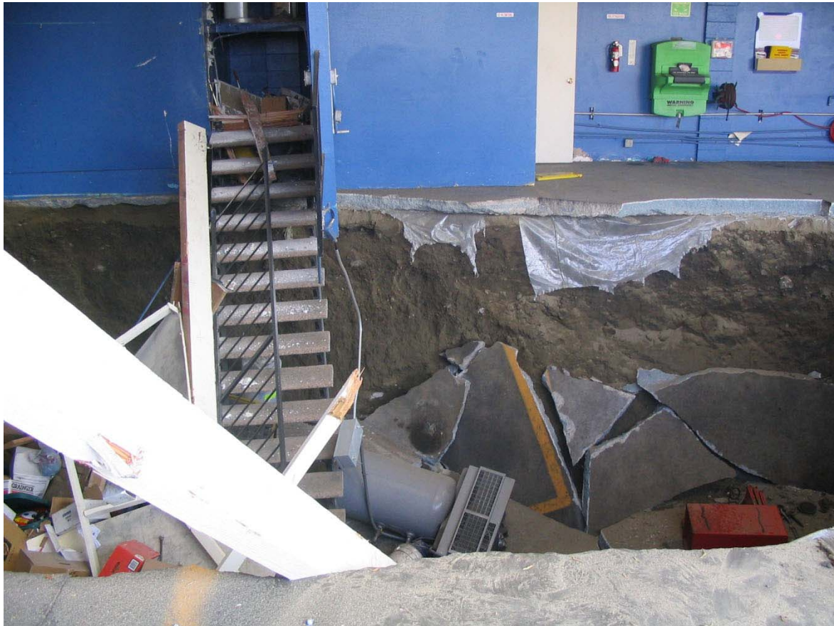
Figure 14: Collapse of the La Cienega Interceptor Sewer under a Building
