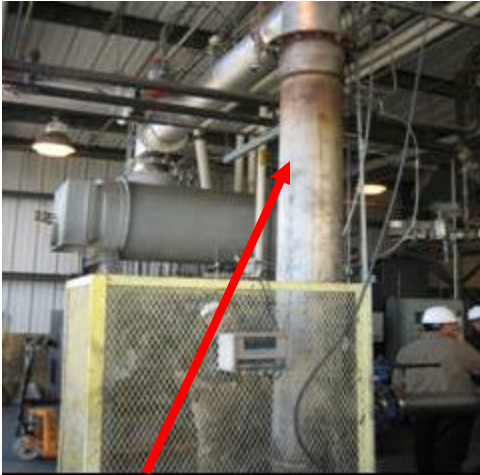
Syngas pipe routed to gas cleaning system
