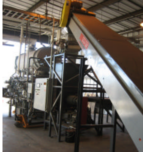
conveyor belt feeds Gasifier
