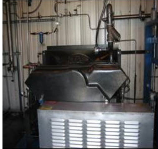
Heat exchanger to recover heat and cool off the syngas
