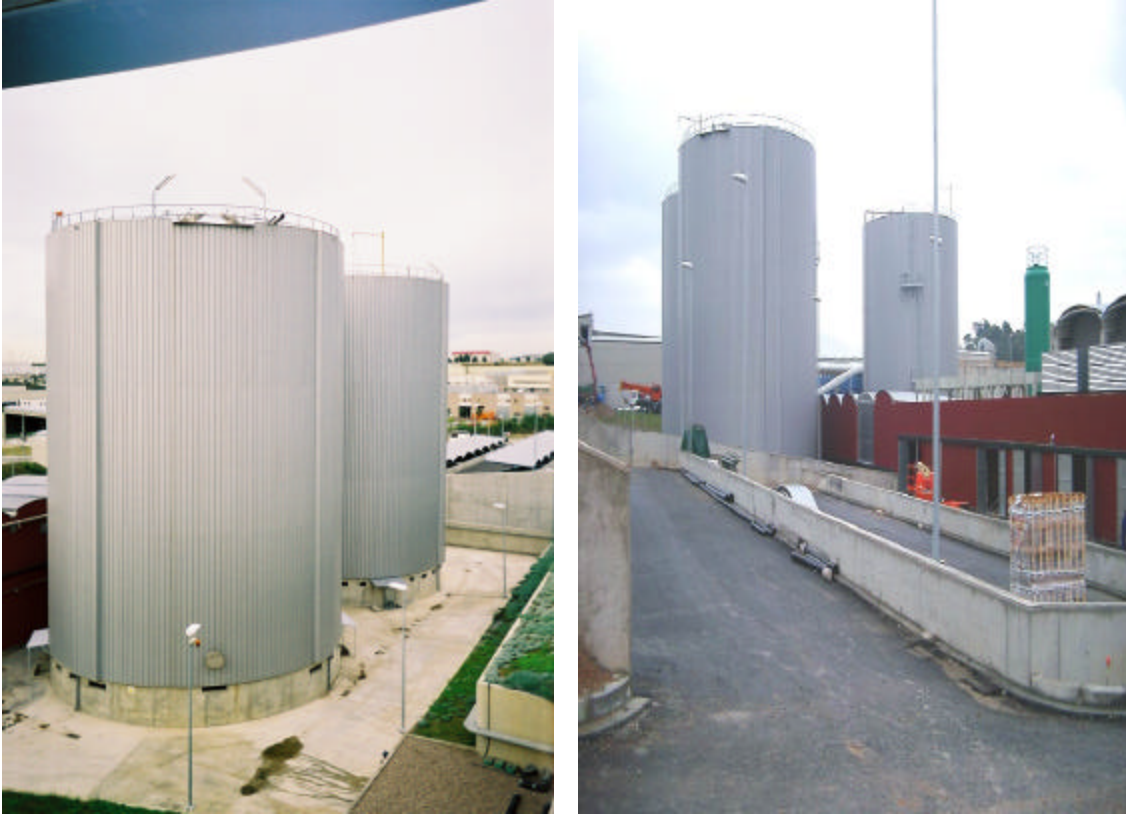
All three Anaerobic Digesters (Valorga Unique Technology)
