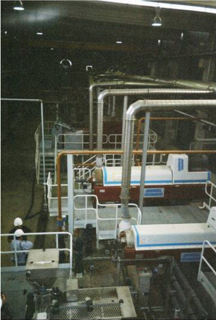
Filtrate centrifuges; screw presses are in the background
