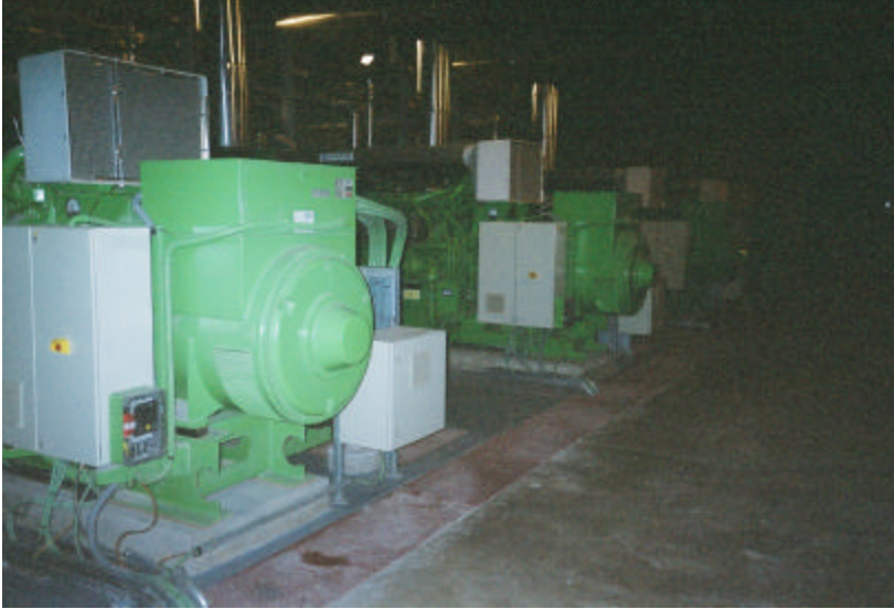
Diesel generators fueled with biogas
