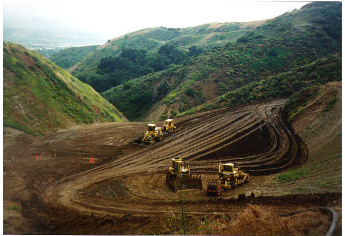
Lopez Canyon - Monofill Construction Toyon Canyon will receive similar closure Estimated completion date 2002
