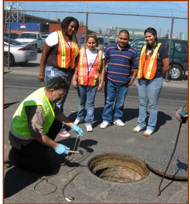
Carolyn Cardenas (right) looks on with Herbert Corleto of CH2MHill (no vest), and La Tanya Moore of Dorsey HS (2nd from left) and Veronica Lopez of Grant HS. Ahmed Ghanem of WESD (kneeling) installs a pressure-measuring device.
